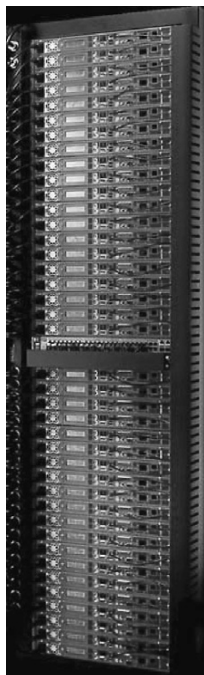
Figure D.19 The TB-80 VME rack from Capricorn Systems used by the Internet Archive. All cables, switches, and displays are accessible from the front side, and the back side is used only for airflow. This allows two racks to be placed back-to-back, which reduces the floor space demands in machine rooms.
